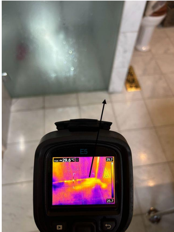
Leaking shower screen identified with thermal imaging
