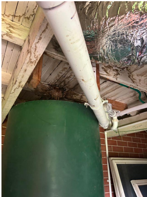
Damages below the shower recess
