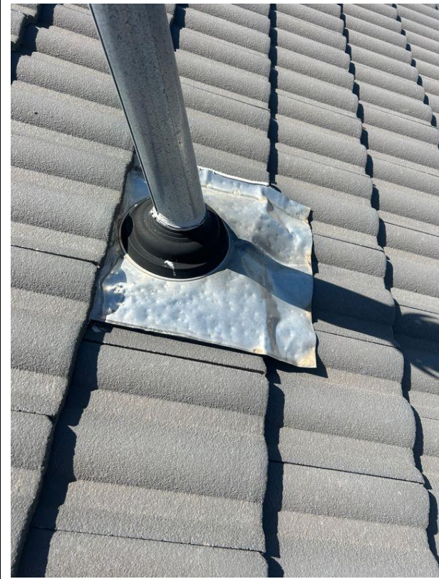
Impact damage identified to the lead flashing
