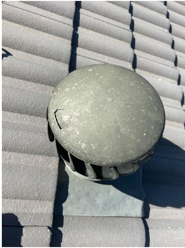
Impact damage identified to the whirlybird
