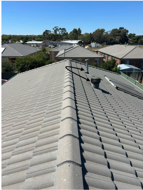
Roof overview and the area of damage
